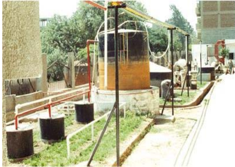
Fig. 5: Biogas digester unit and gas collection [8]
