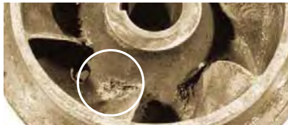
Cavitation corrosion of bronze impeller
