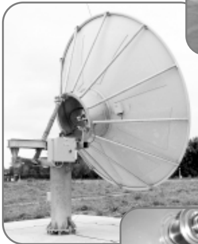
Satellite Dish Positioning
