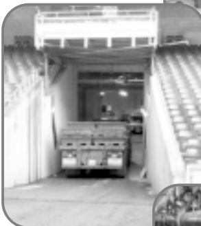
Stadium Access Lift
